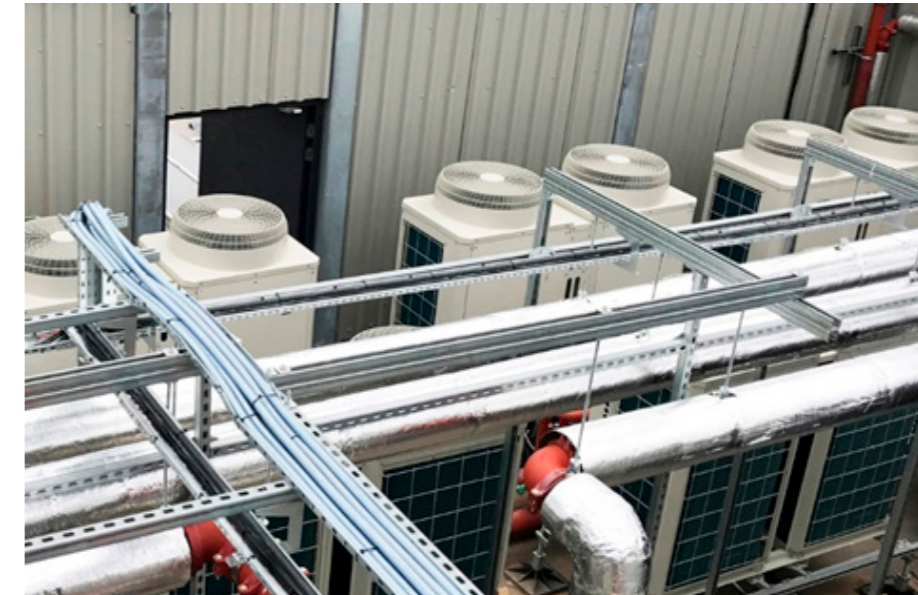
Figure A.56: Air Source Heat Pumps
